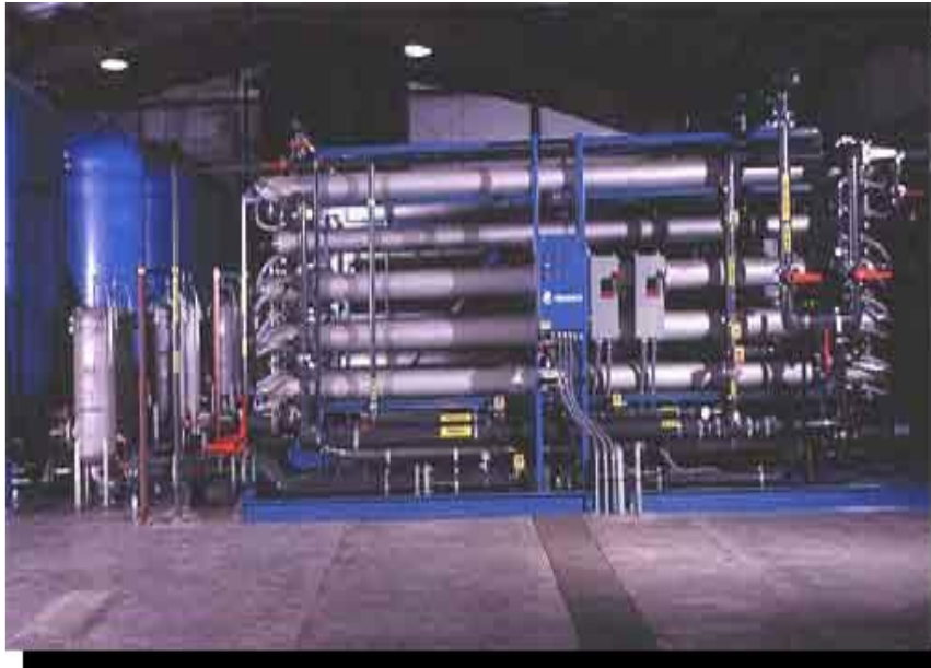
Reverse Osmosis System
